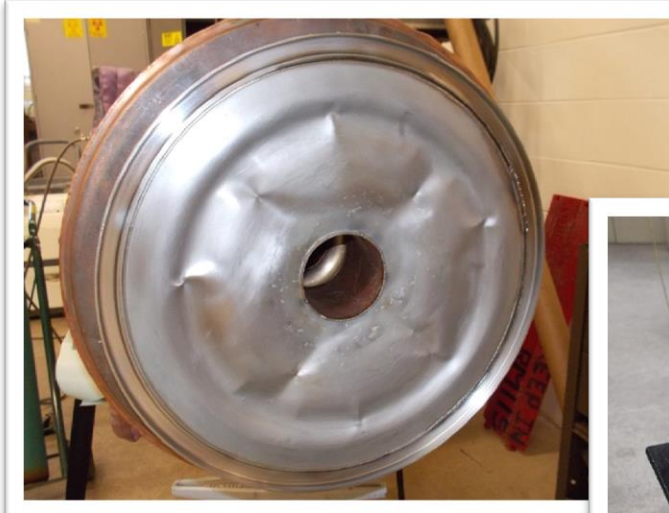
Leaking “pie-tin” quick disconnect flange
