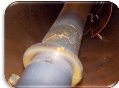
Internal sparking and damage
